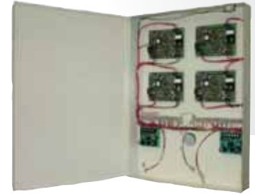
8-door controller (large cabinet)
