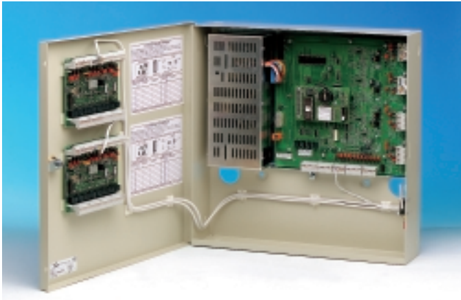
Alarm Controller showing two AEMs mounted inside the cover
